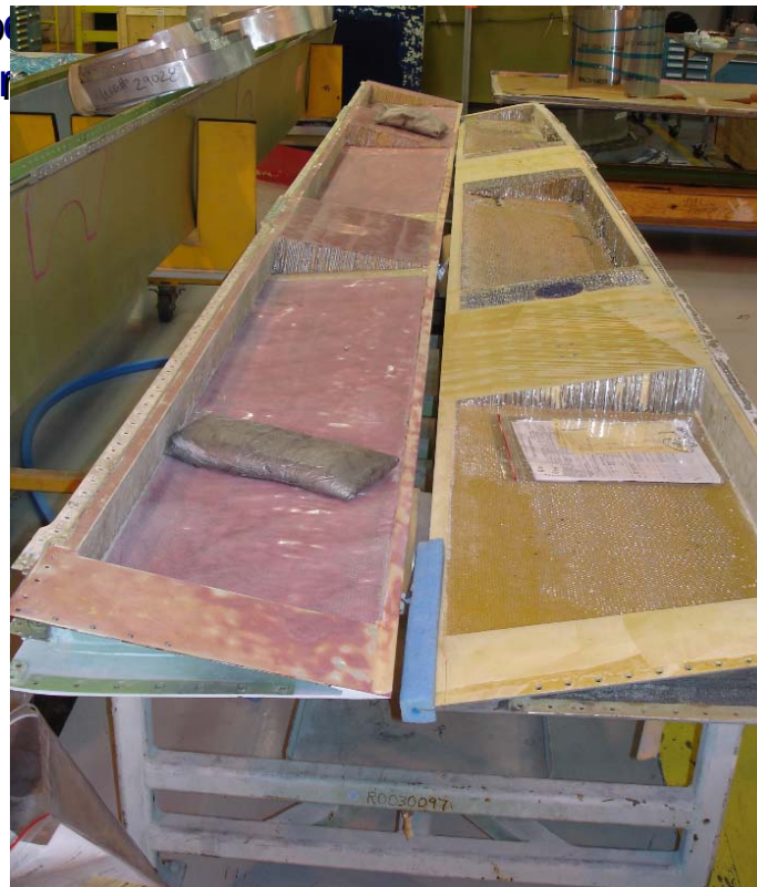
Airline Perspectives on the Constraints of Bonded Repair Size Limits
