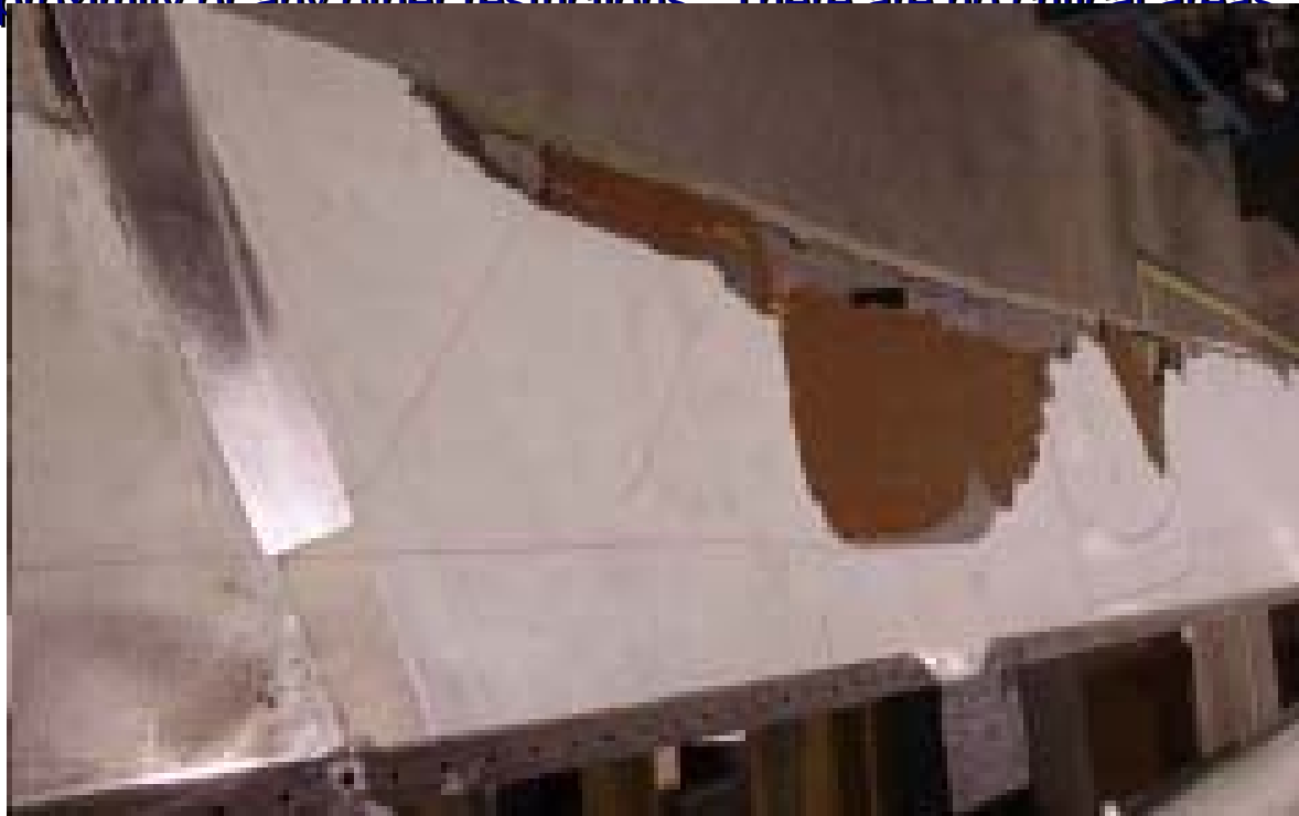
Airline Perspectives on the Constraints of Bonded Repair Size Limits
